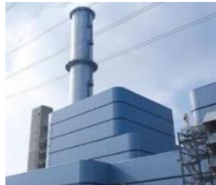
SGT5-8000H (intro) CCPP Irsching 4 1S / 578 MW
